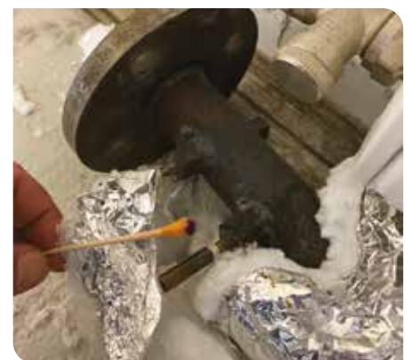
Cr VI found within insulation
